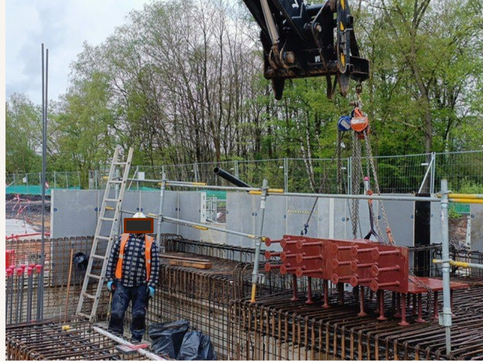
Placement of steel inserts for the mounting of the moving floor Tolerance +/-1mm
